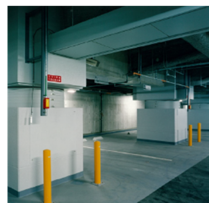
Quake-absorbing equipment installed (1st basement floor)
